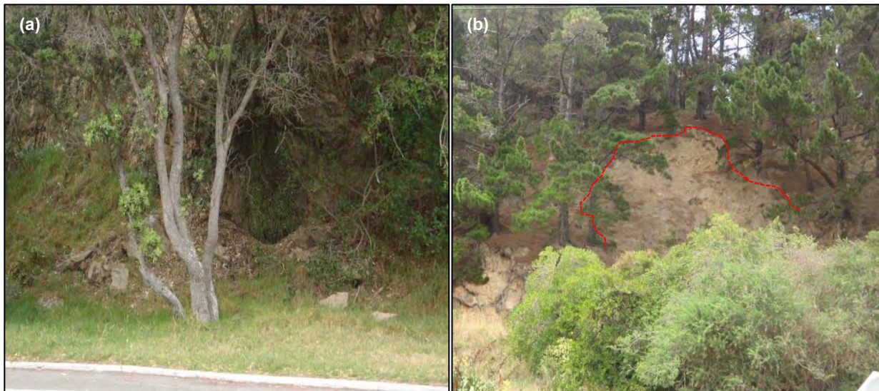
Figure 6 (a) Rock fall debris at toe of Slope 5; (b) Extent of shallow surface failure above greywacke outcrop at Slope 8
