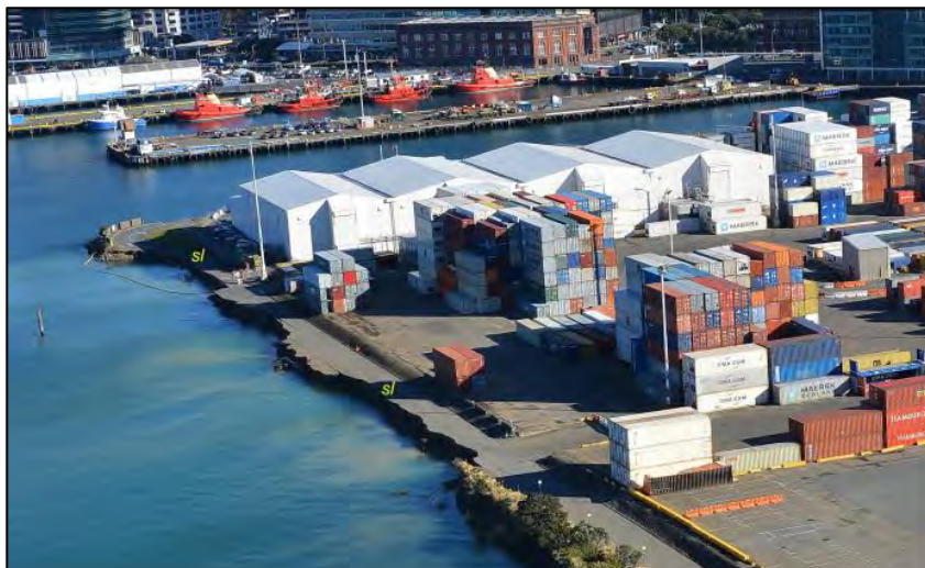
Figure 4 Effects of Liquefaction and Lateral Spreading upon Quayside Wall, Wellington, 2013 (Ref. 9).
