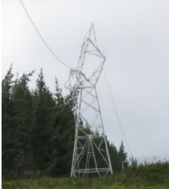
Photo 2: Damage to the Bunnythorpe-Wairakei A transmission line caused by plantation forestry falling into the line. The damage was caused by plantation forestry falling into the line near Rangipo in 2012. New foundations and tower repairs were in the order of $500,000.
