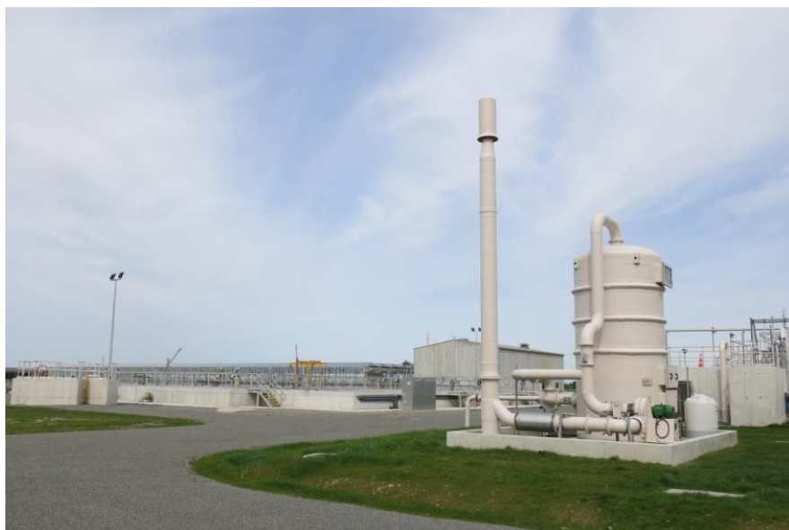
Photo 5: Biological scrubber at wastewater treatment plant
