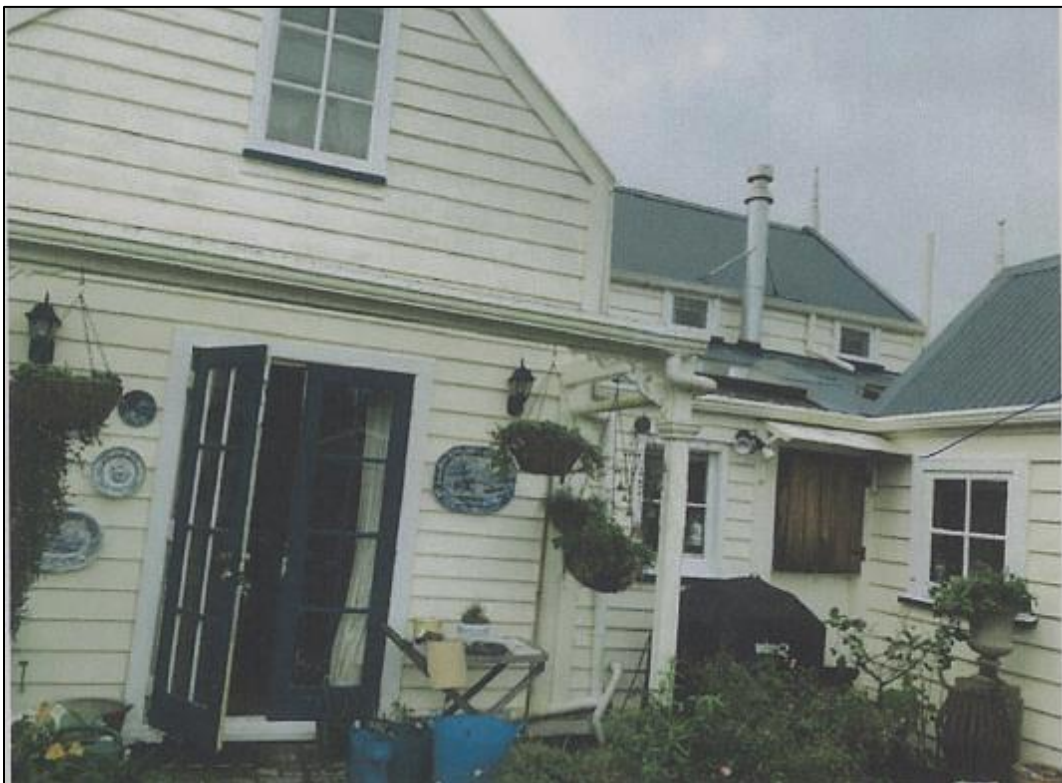
Rear western elevation. Note the buttery door to the right of image (Hawley, 2001).
