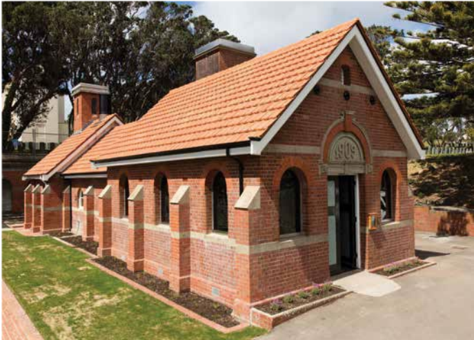
The Karori Cemetery Chapel was strengthened in 2016 in a sensitive scheme that preserves both the original use and structure.
