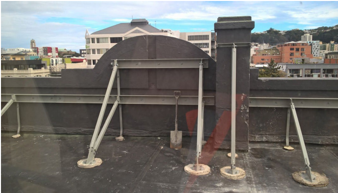
New structural elements to secure the existing parapet and chimney at the former Cadbury Building has been installed so that it is not visible from Ghuznee Street. (Photo: Wellington City Council, 2018)
