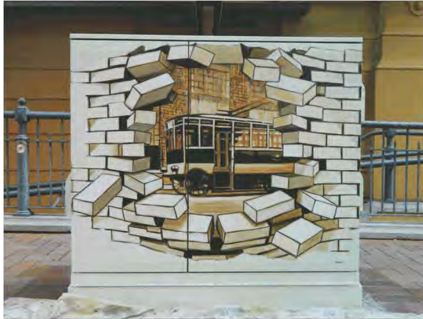
Figure 4: TBOP Electrical Fault Protection Cabinet in Pigeon Park, Te Aro
