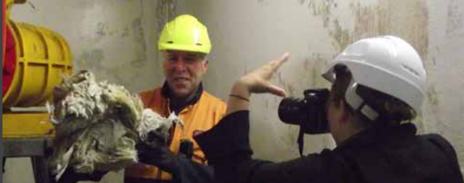
Hutt News reporter Karoline Tuckey grabs a picture of Hutt Valley Water Services' Steve Daken holding what's blocking the pumps at wastewater pumping stations.
