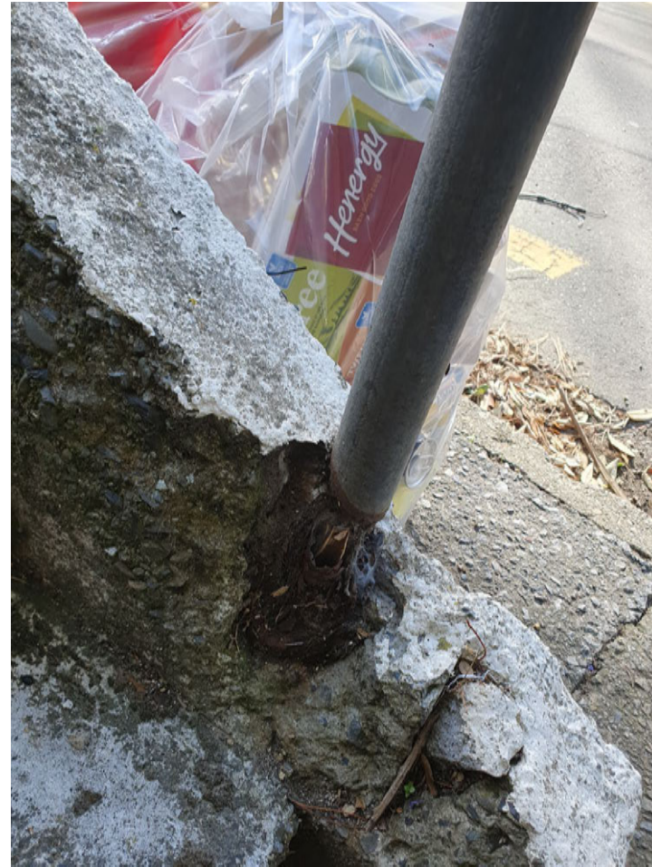
Metal post with railing to steps to 72-76 dislodged from concrete base by reversing trucks etc
