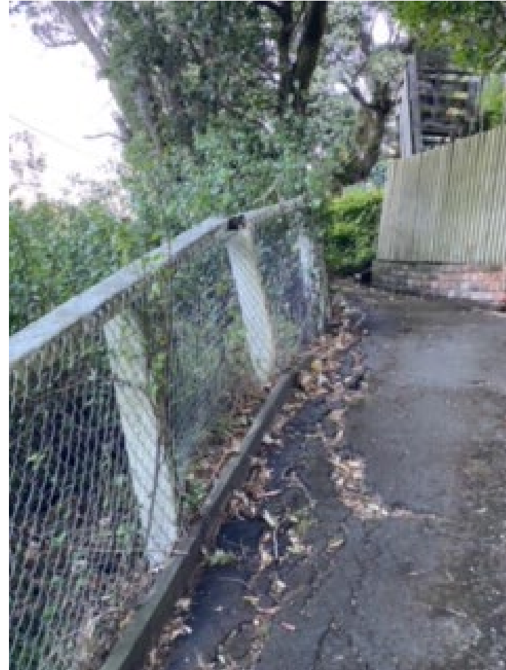
cracks in path
