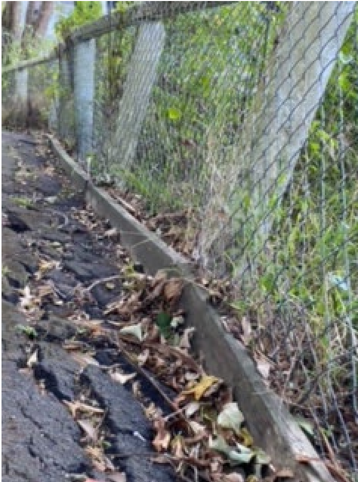
Cracks in ground by handrail
