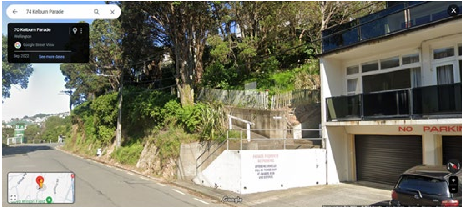
Kelburn Parade steps built when WCC gave consent to build drive-on flats in front of 70KP. Railing on steps leading to 72-76KP dislodged from concrete base.
