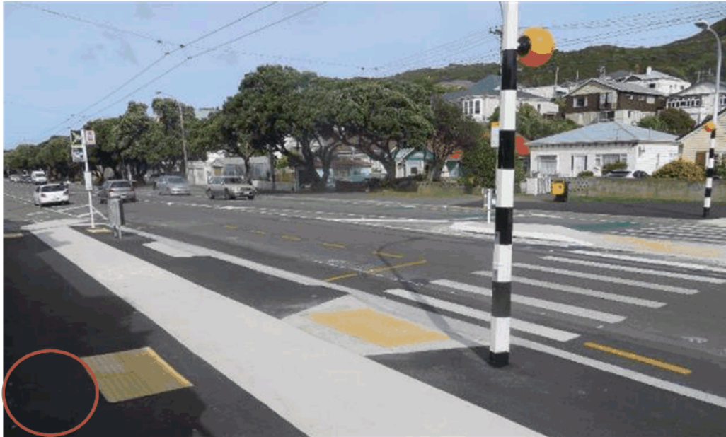
Figure 2-26: Photo showing missing directional tactile pavers on the eastern side of the pedestrian zebra crossing located south of Dee Street.
