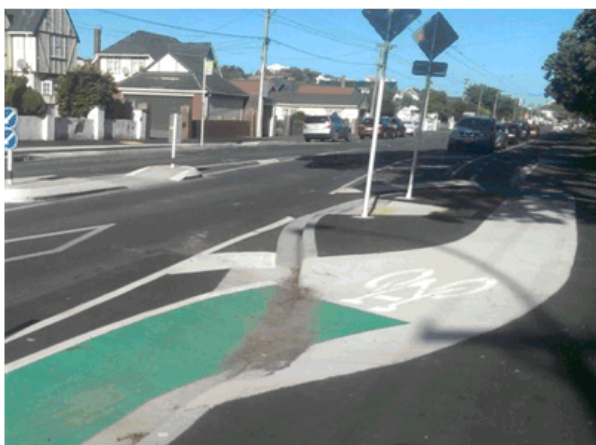
Figure 1: Surface water and debris pooling at cycleway transition
