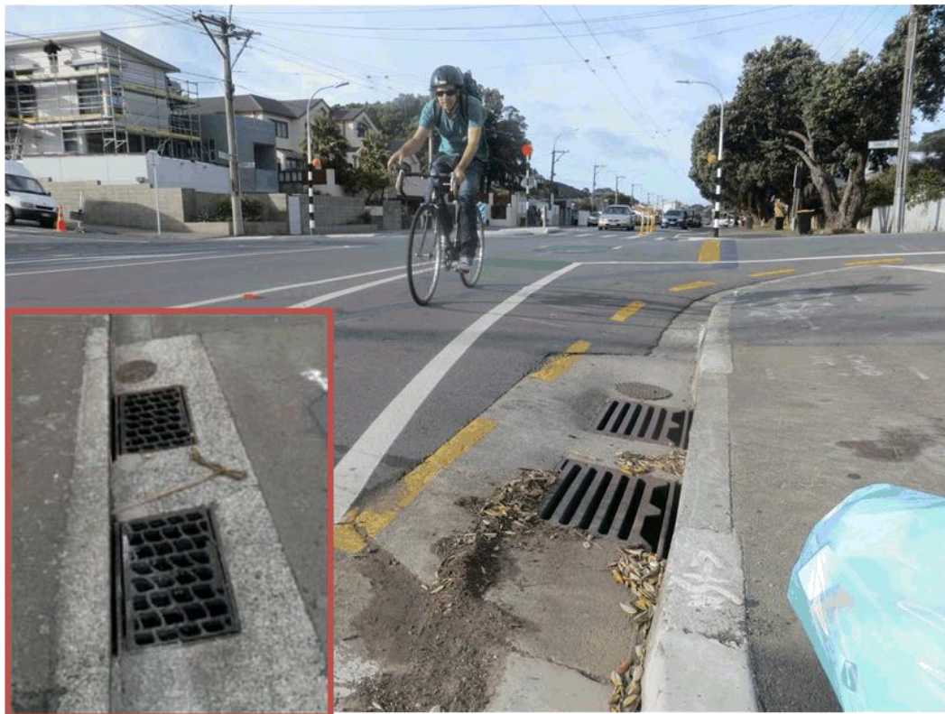
Figure 2-18: Photo showing a non-cycle friendly sump at Tamar St/The Parade (inset photo: example of cycle friendly sumps elsewhere along the route).
