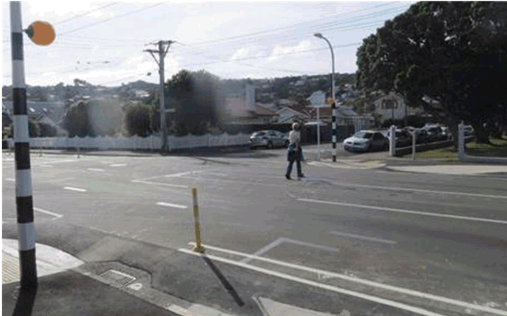
Figure 2-20: Photo showing the partially built pedestrian zebra crossing south of Humber St
