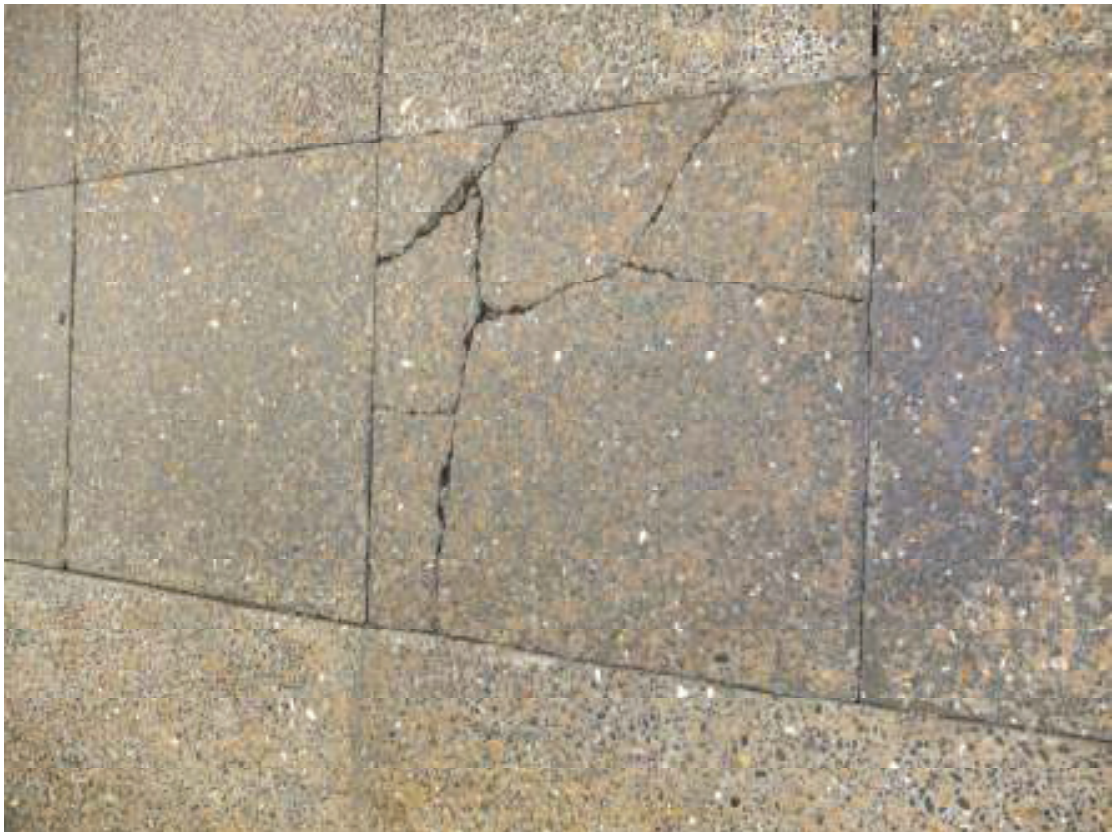
12 broken paving under the canopy
