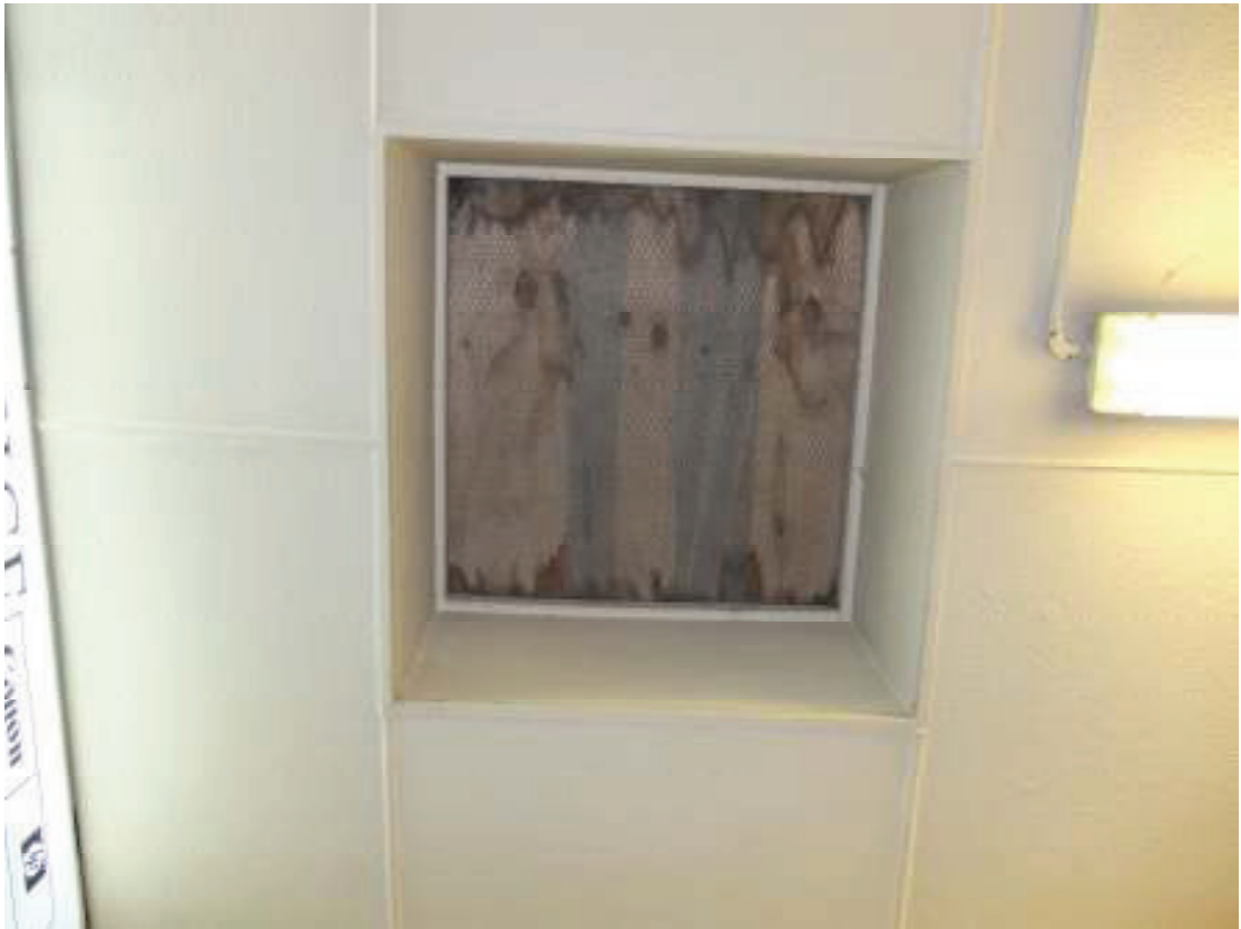
11 plywood covering canopy's former Perspex skylights
