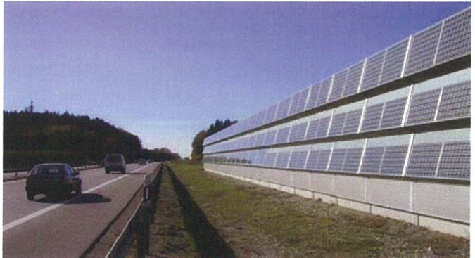
PV system mounted on a noise barrier
