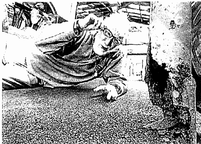
Don McDonald is concerned at the state of some of Newtown's decrepit verandas and awnings, fearing someone could be injured or killed if one collapses.
