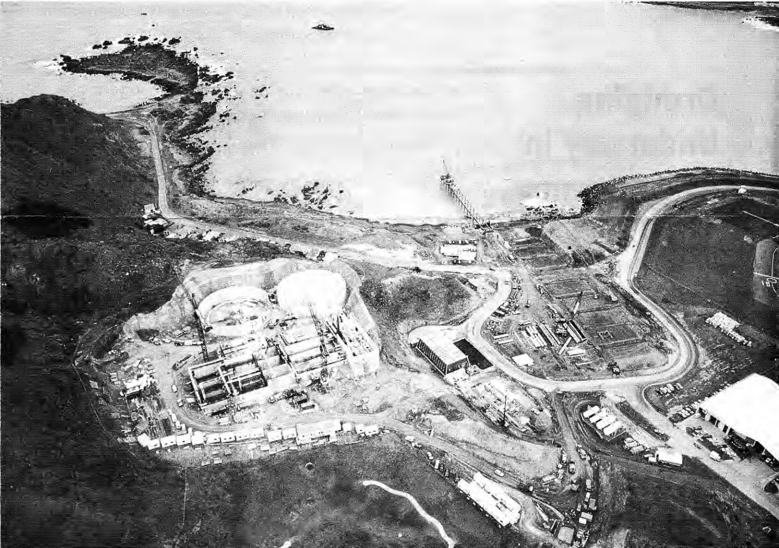
Aerial view of Moa Point construction site extending to barge working on outfall trench John Cheese Photography
