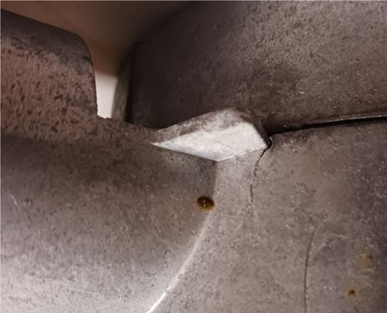
Figure 13 - Right loading Crack Initiation
