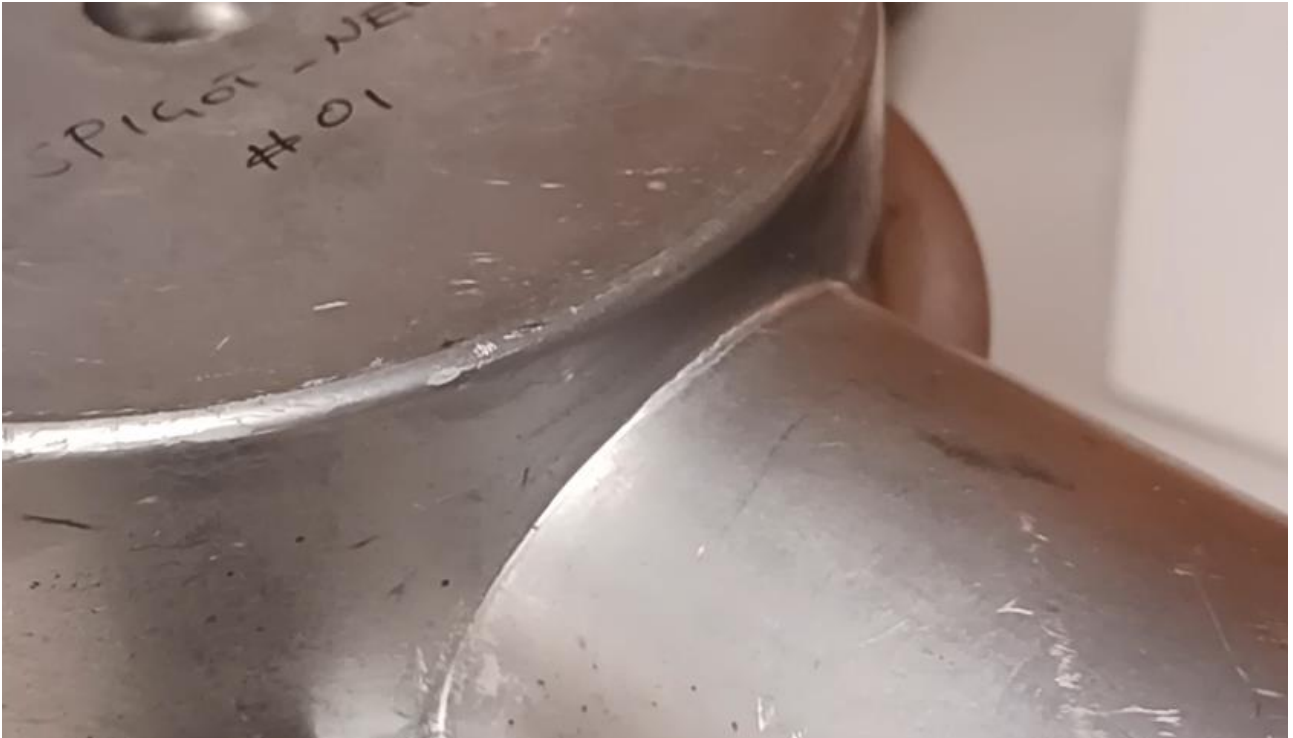
Figure 15 - New spigot - Crack initiation
