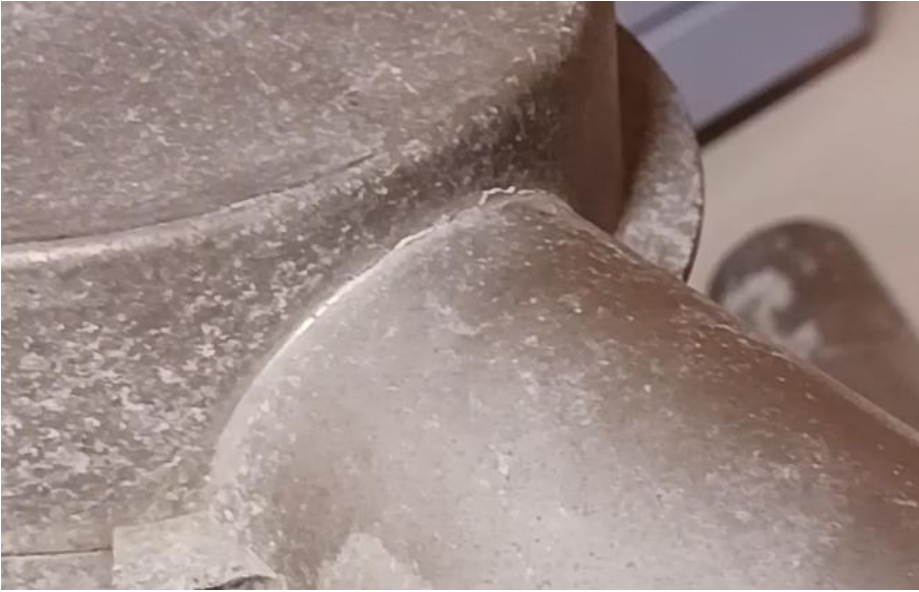
Figure 9 - Left loading Crack Initiation
