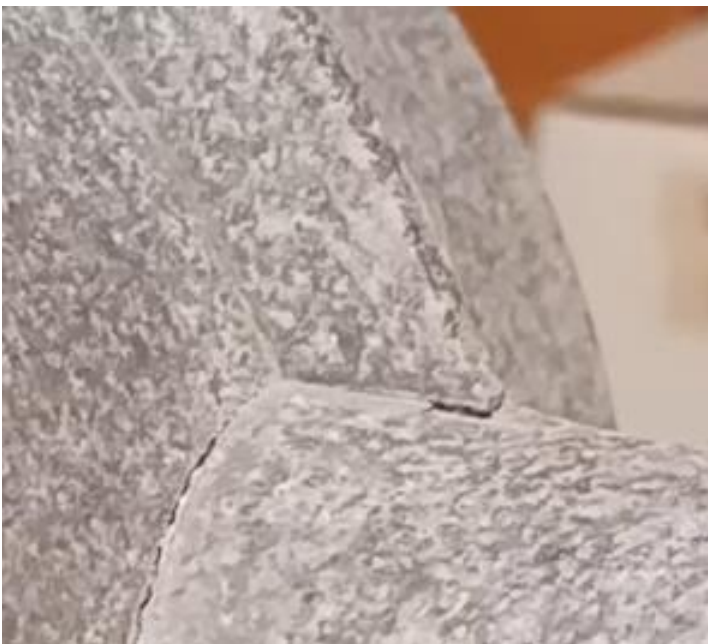
Figure 6 - Vertical Load Crack Initiation
