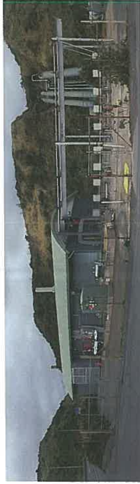
WELLINGTON WATER PUMP STATION, BORE DRAIN AND GUTTER PROPOSED TO BE INCORPORATED INTO DISPOSAL PIPES AT RIGHT, LINK WITH UPPER WINTAR TREATMENT PLANT.
