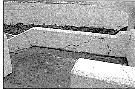
Cracked concrete wall
