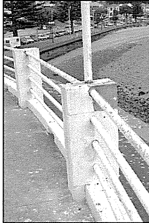
Rusting steel balustrading causing spalling concrete
