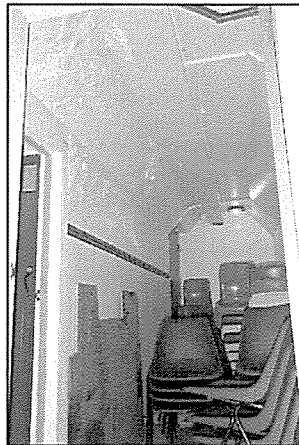
Efflorescence and spalling plaster
