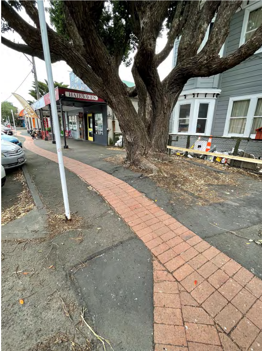
Poor accessibility with path at an angle and cracked
