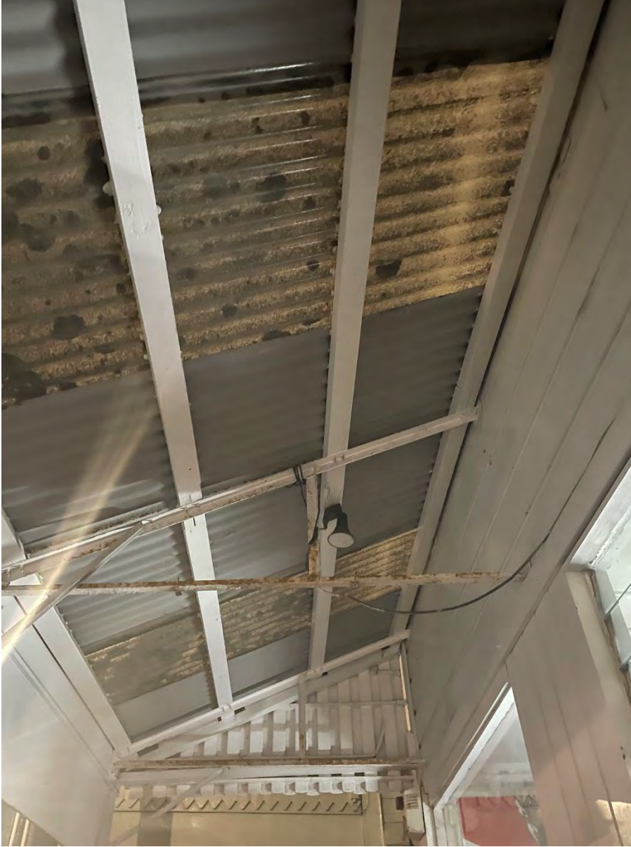
An example of under canopy lighting not in use
