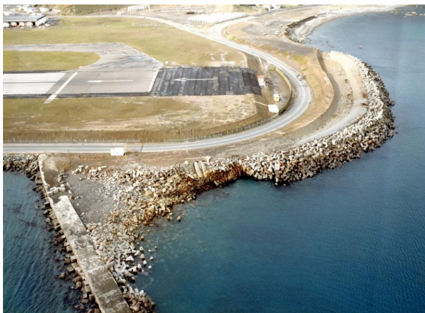
Photo 8: June 1983 seawall breach
