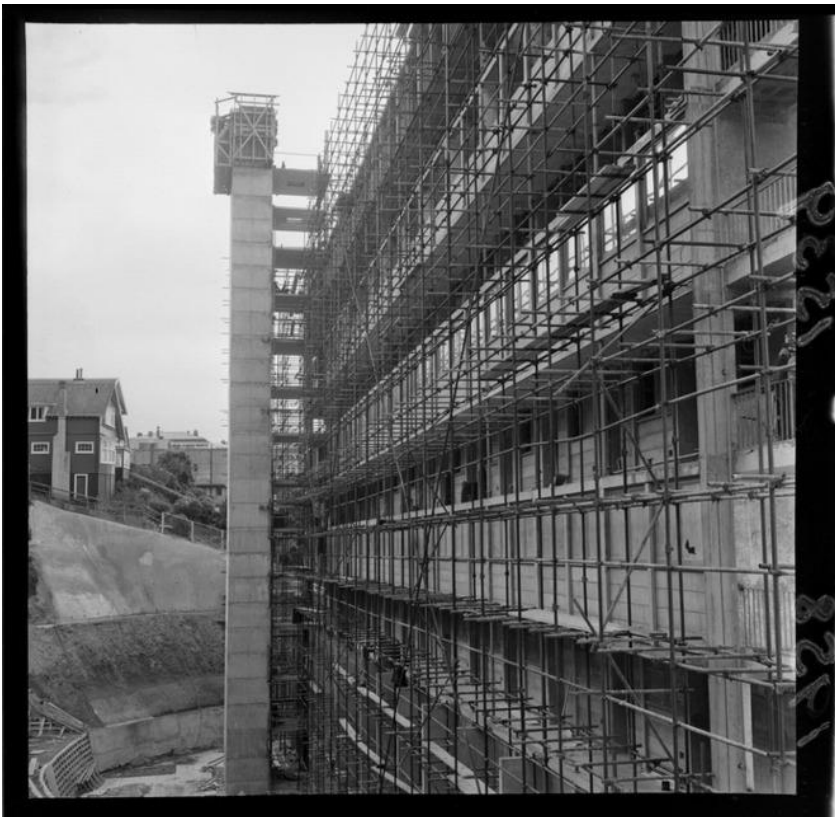
Figure 6: [Gordon Wilson Flats], Construction of lift tower, 1958. EP/1958/1539-F, Alexander Turnbull Library, Wellington.
