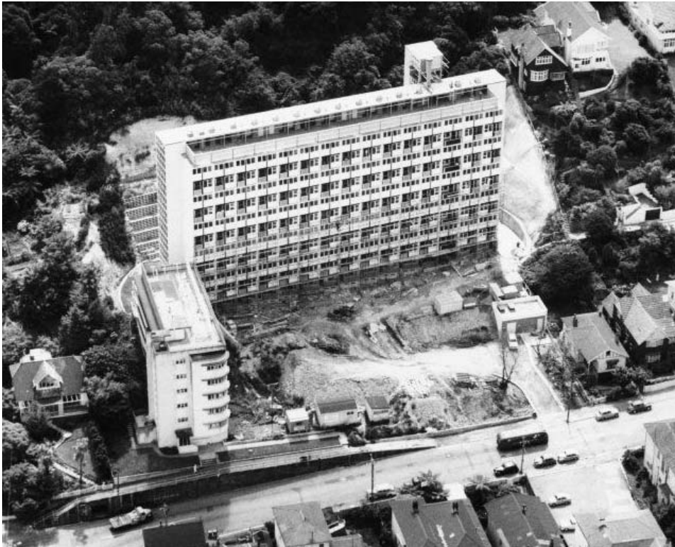
Aerial view of the Gordon Wilson Flats under construction c1958-9. The McLean State Flats are to the left (Ref: EP-Industry-Housing-State-02, ATL)
