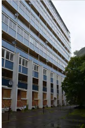
Figure 22. Looking south along the western elevation. Note the slender buttresses that act as stiffening members anchoring the structure to the pile heads. (Archifact-Architecture & Conservation Ltd., 2014)
