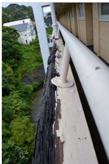
Figure 70. Looking at the extent of decay apparent in the balcony balustrading. (Archifact-Architecture & Conservation Ltd., 2014)
