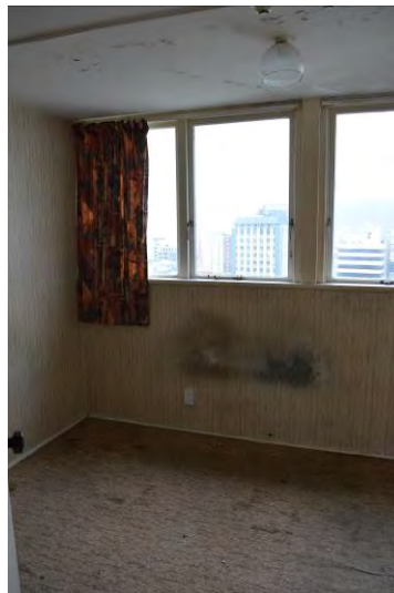
Figure 57. Looking at a typical east side bedroom. Note damp patch with mould growth on the external wall. (Archifact-Architecture & Conservation Ltd., 2014)
