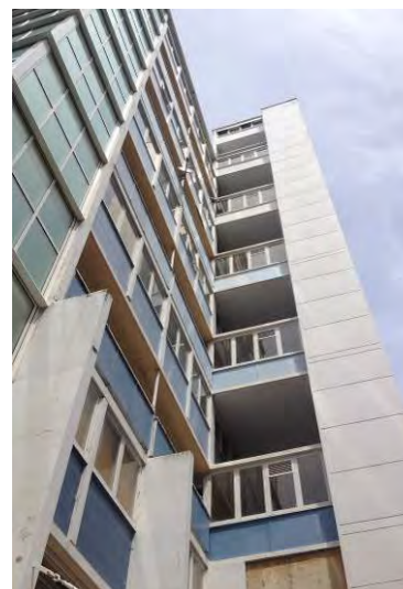
Figure 20. Looking south towards the lift tower and its junction with the west elevation. (Archifact-Architecture & Conservation Ltd., 2014)
