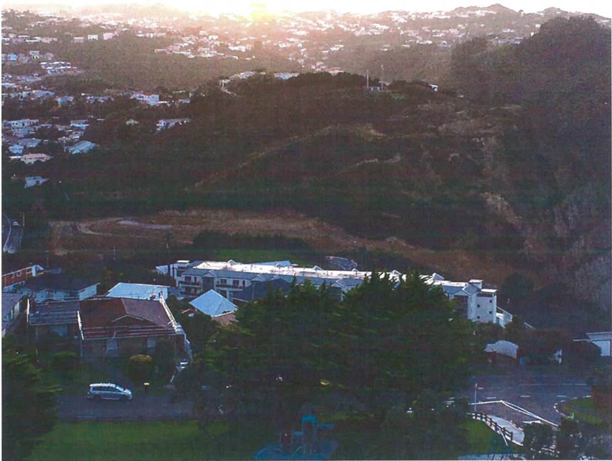
Image 2: The view towards Raroa when significant earthworks and further slurry dump has been created.
