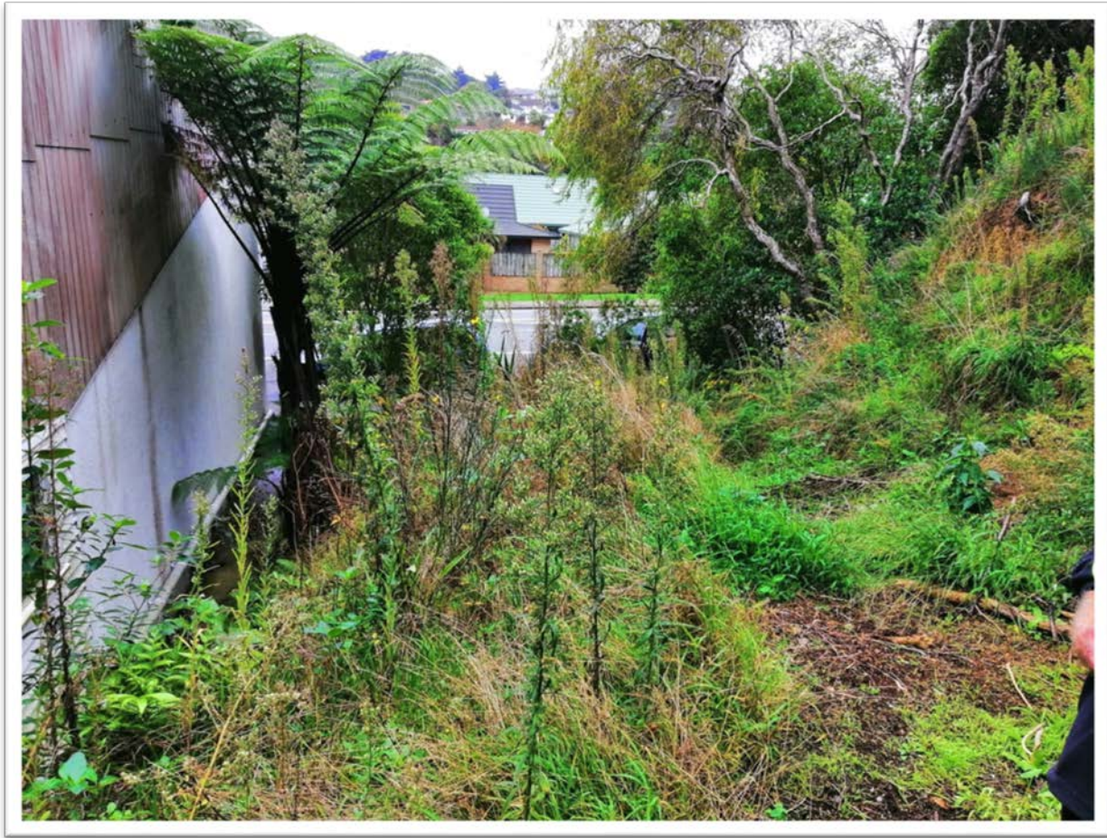
Photo 4: west side of clubrooms facing east illustrating the area to be excavated
