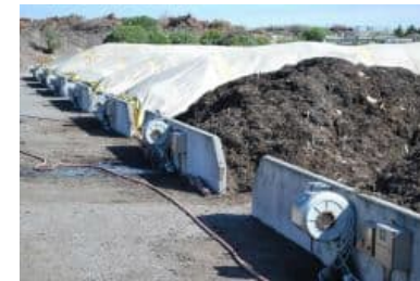
Figure 5-1 Timaru composting facility
