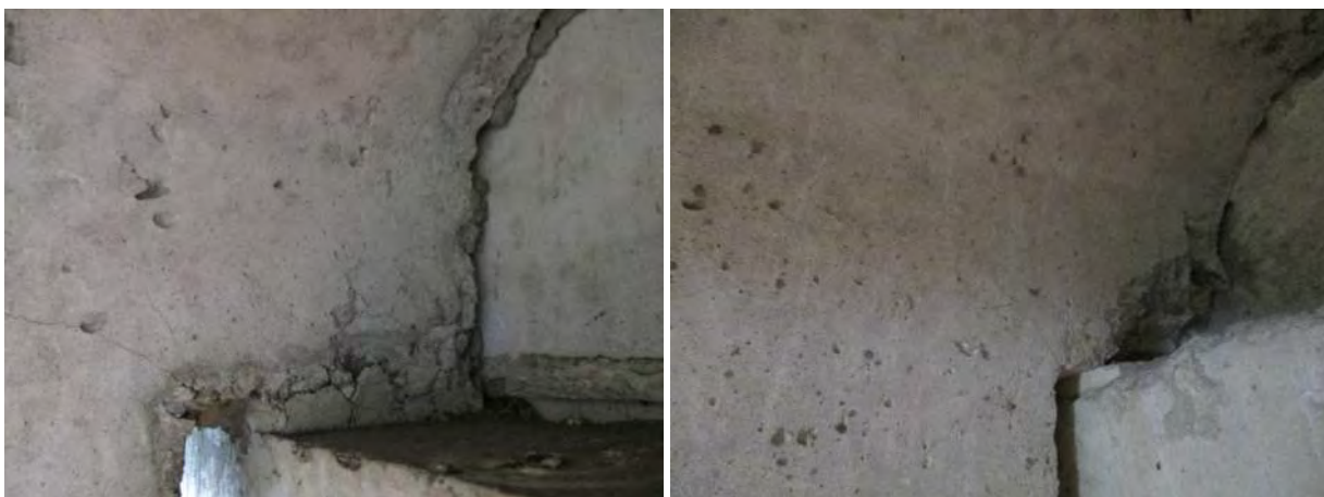
Figure 8 - Double tee support conditions - (Left) double-tee units positioned directly against the beam and (right) initial spalling at the back of the double-tee unit
