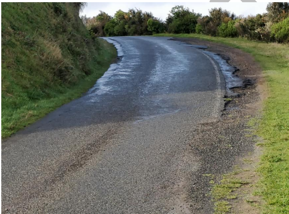
Figure 4-2: Typical example of edge break seen in Section B
