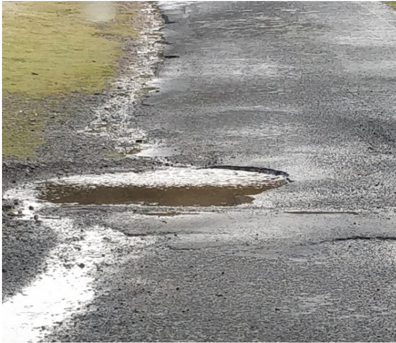
Figure 4-7: Large pothole requiring repair in Section D
