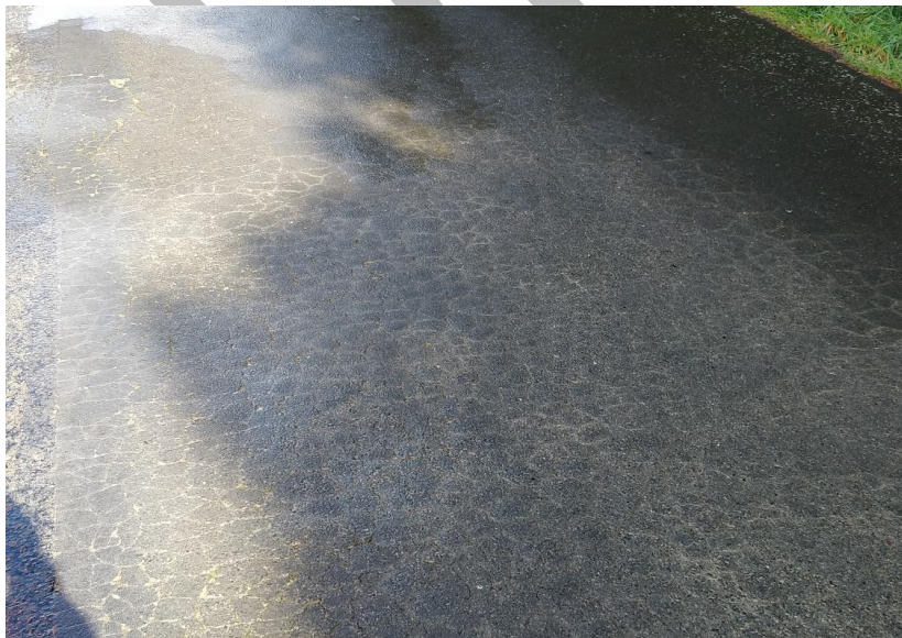
Figure 4-1: Area of failed AC with crocodile cracking evident
