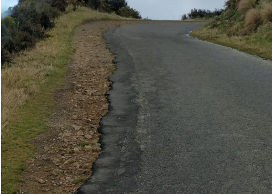
Figure 4-6: Typical view of edge-break in Section C
