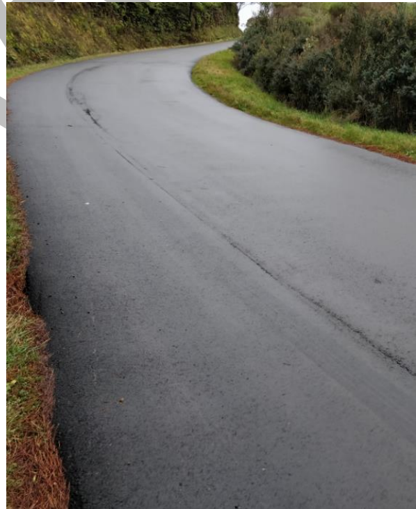
Figure 4-5: Recent AC pavement repair on Section B (Near Southernthread Road)
