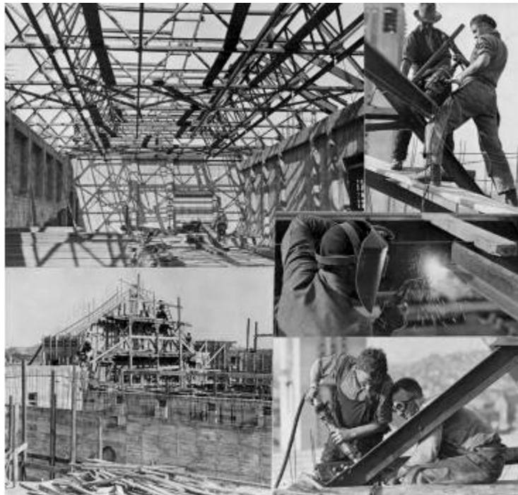
Montage of images showing the Dominion Museum under construction, Buckle Street, Wellington. Negatives of the Evening Post newspaper. Ref: 1/4-015181-F. Alexander Turnbull Library, Wellington, New Zealand. http://natlib.govt.nz/records/22740117
