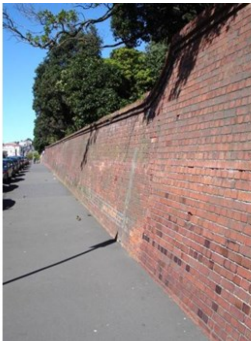
Tasman Street Wall. Copyright: NZ Historic Places Trust. Taken By: Michael Kelly. Date: 1/10/2007.
