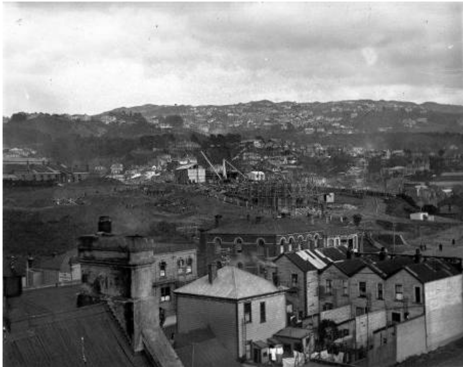
Carillon under construction. Negatives of the Evening Post newspaper. Ref: 1/2-090208-G. Alexander Turnbull Library, Wellington, New Zealand.
