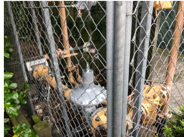
Photograph 4: Utility Gas Junction Located Adjacent to the Northeast Portion of the Property.
