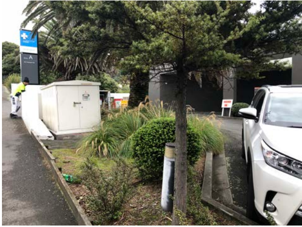
Photograph 5: Transformer Located Adjacent to the Property.
