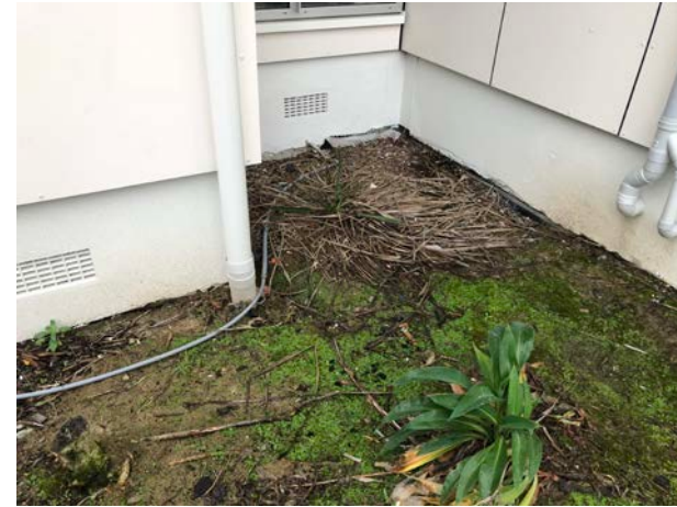
Photograph 8: Deteriorating Paint Along Base of Building.
