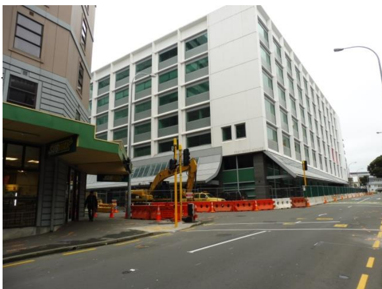
PHOTO 1: Defence House (Ministry of Defence) demolished following November 2016 Kaikoura earthquake
