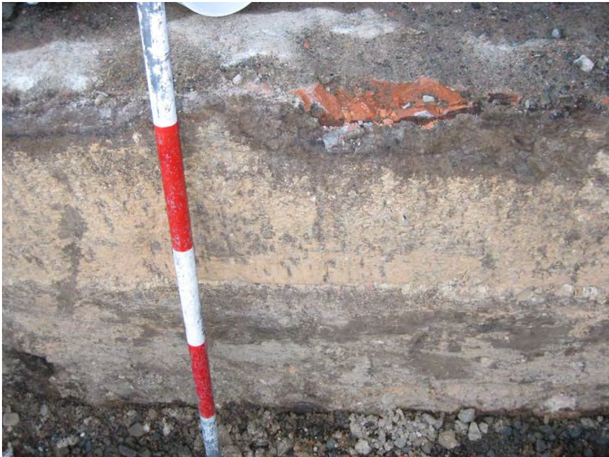
Figure 20: Detail view of tanking (bitumen cast behind boxing?) against brick of the Customhouse foundations.
