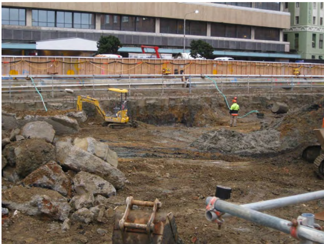
Figure 18: General view, looking west. Exposed seawall in centre of image, immediately to right of digger O'Keeffe
