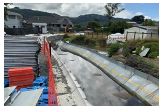
Retaining wall and stream divider as part of the Pinehaven Stream Improvement
