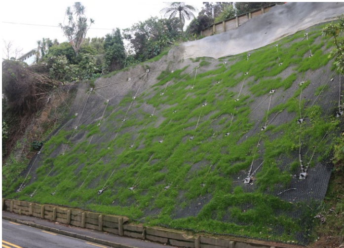
Slope stabilisation on Lennel Road in Wadestown erosion netting, anchoring and spraying of shotcrete
