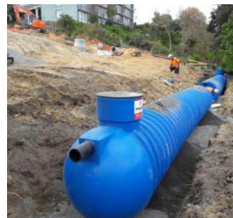
Underground stormwater tank installed as part of land development
