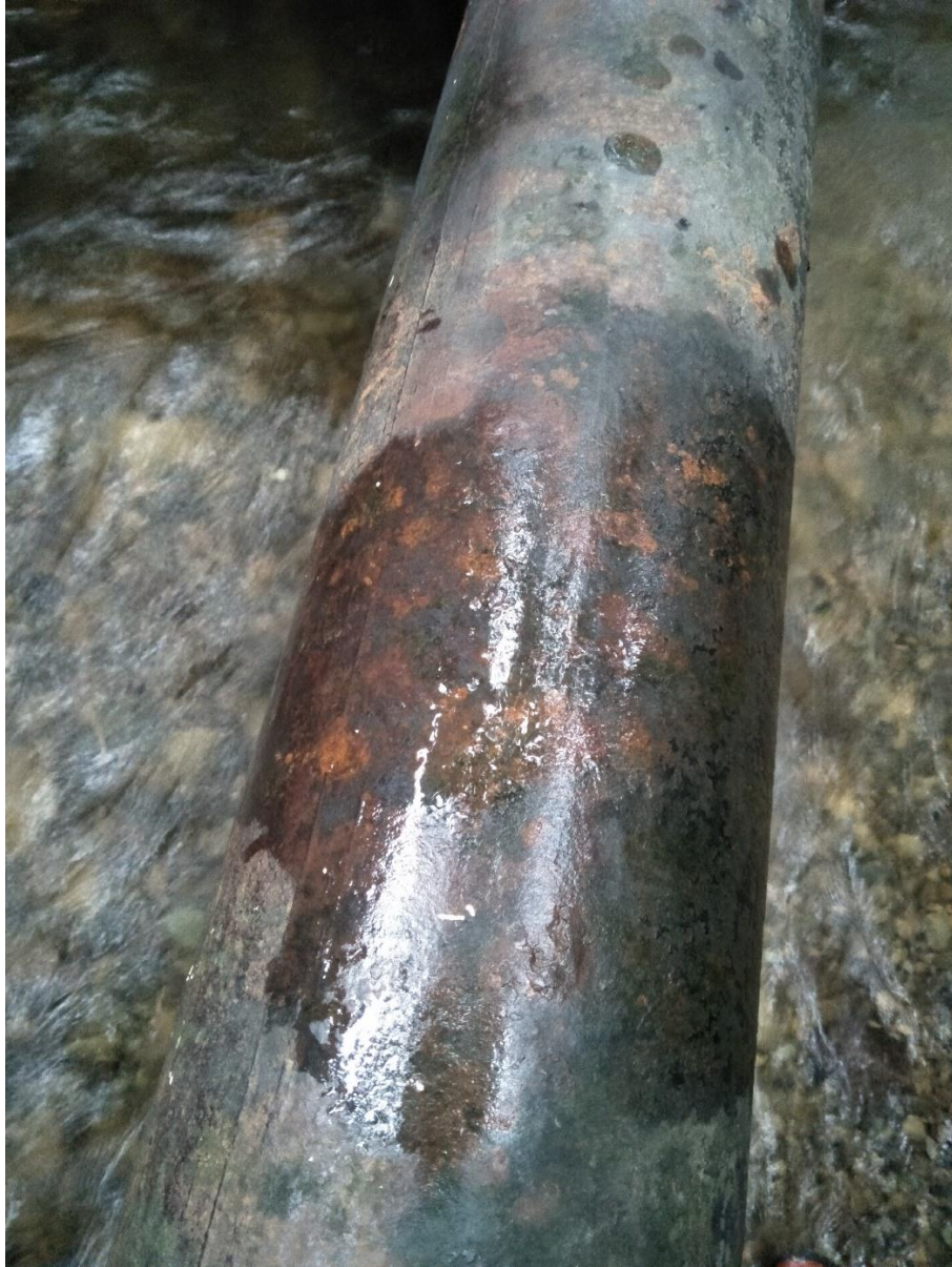
Seepage out of a cast iron waste water pipe over Tyers Stream
