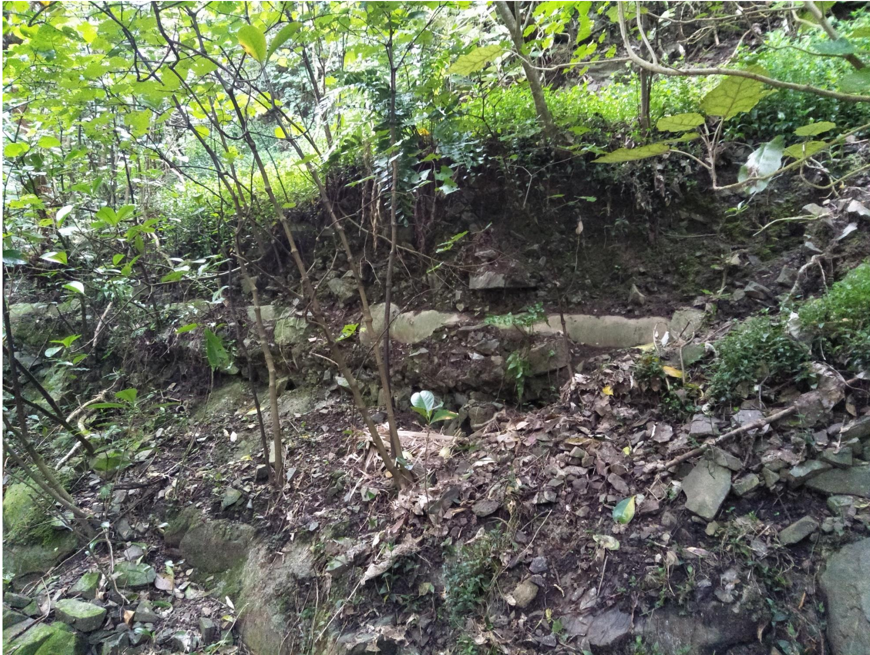
Waste water pipe in Tyers Stream Reserve exposed due to erosion. If it fails it would be difficult to fix rapidly due to poor access and unstable slopes
