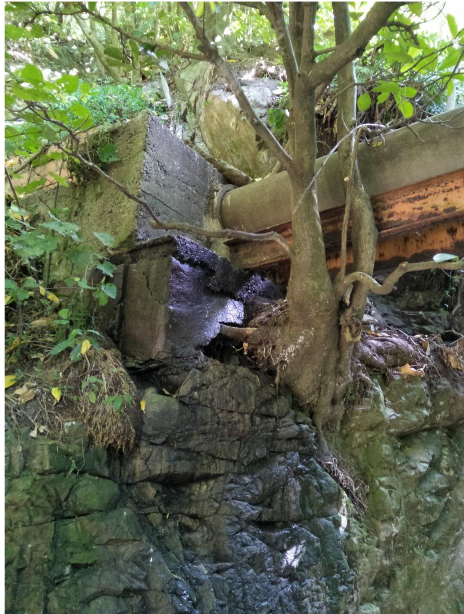
Leaking wastewater pipe collar over Tyers Stream, leaking on and off since April 2021.
