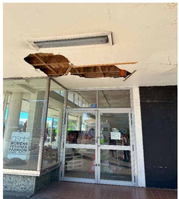
Main Street building decay. Gladstone Rd
