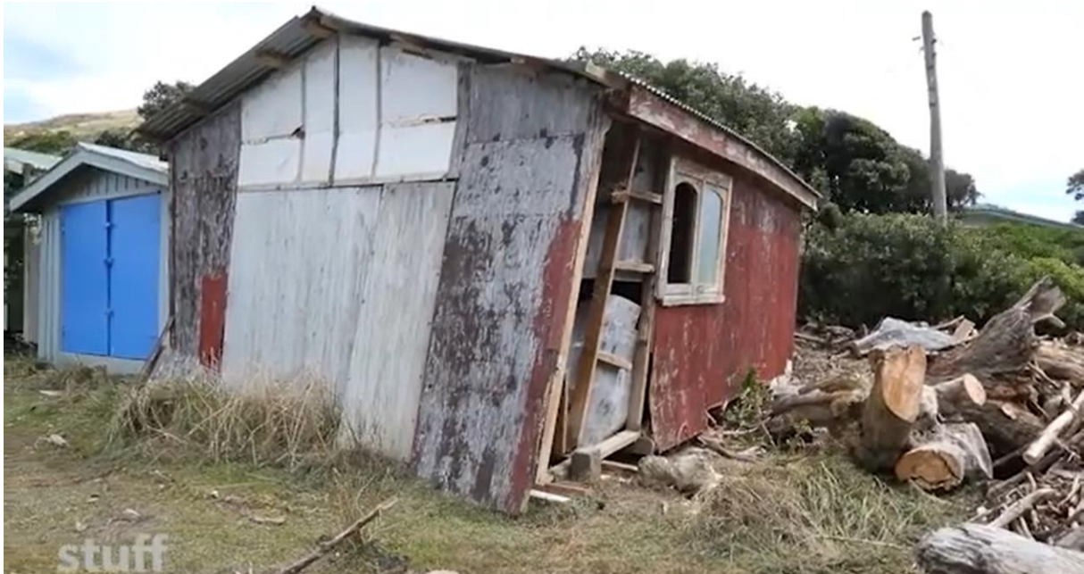
Figure 6-36: Validation site 3. Here the water levels were significantly higher as can be seen from the damage to the boat shed. https://www.stuff.co.nz/environment/110423337/wellington-seaside-village-hatches-climate-change-plan-after-cyclone-gita-mayhem .
