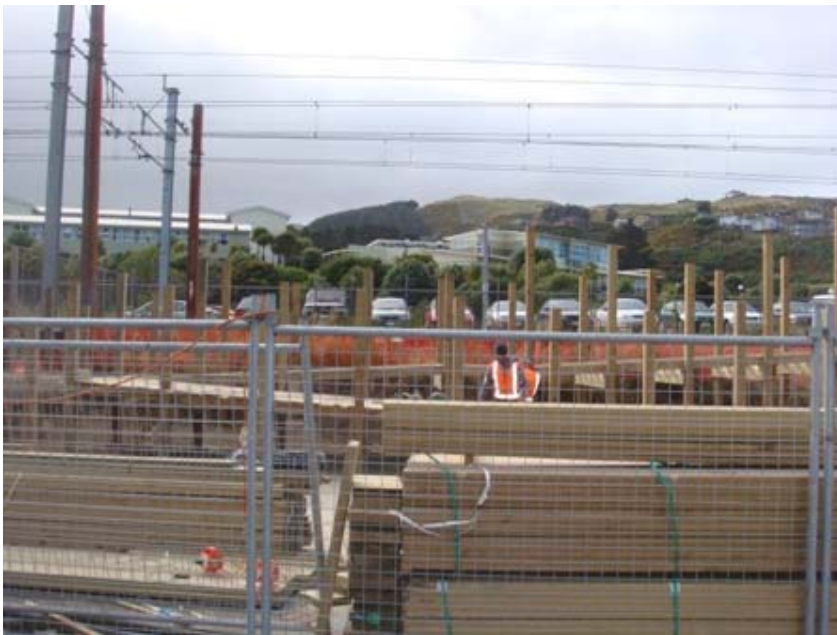
Progress on the access way across the railway tracks. Completion expected in July.
