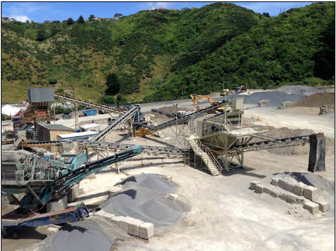
Figure 1-5: Photograph of the Kiwi Point Quarry Processing Plant at its Existing Location
