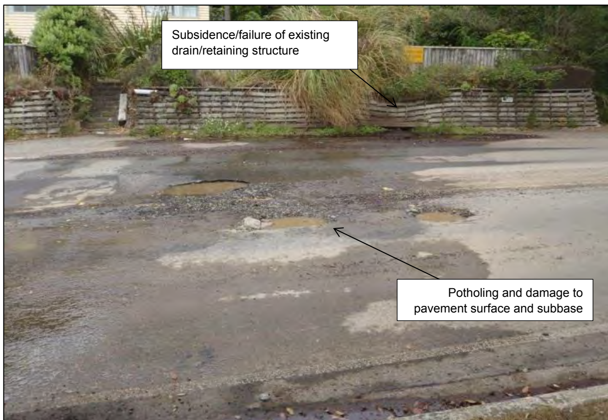
Figure 10 Road damage due to surface water from gully runoff
