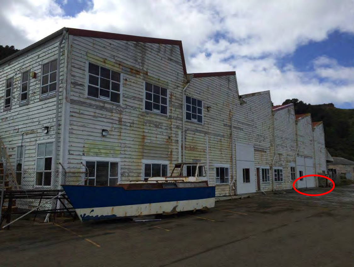
Photo 1. Western side of Shed 8. Photo taken from wharf. Area with critical foundations marked in red.
