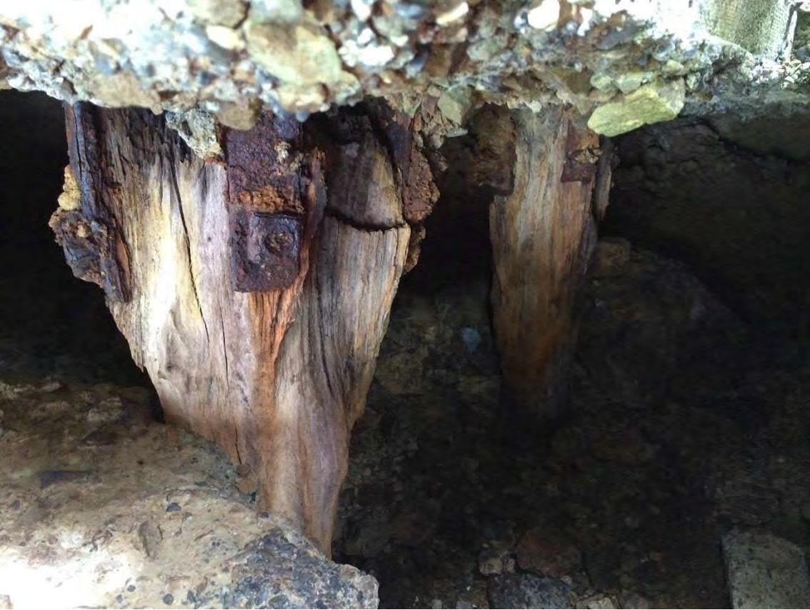
Photo 3. Damaged timber piles – critical foundation No. 1
