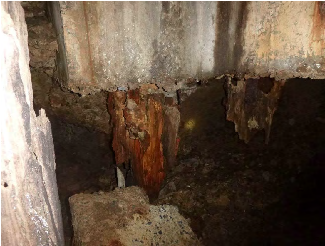
Photo 5. Damaged timber piles – critical foundation No. 2.
